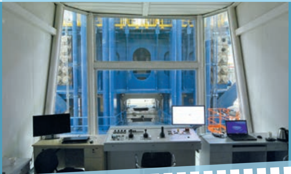
Control room for 500 MN press
