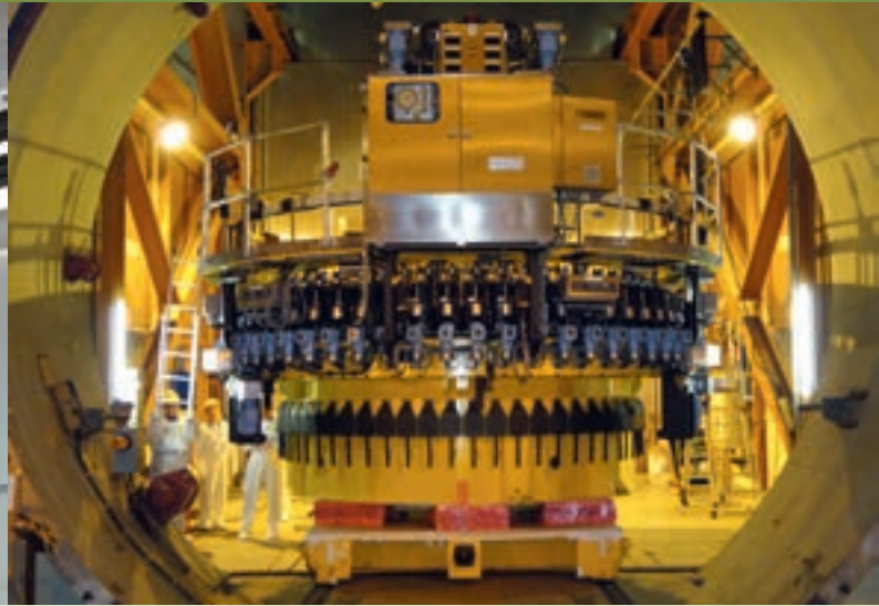
Nuclear power plant Gravelines 2011: Transport of a multi stud tensioning machine through the material lock into the containment
