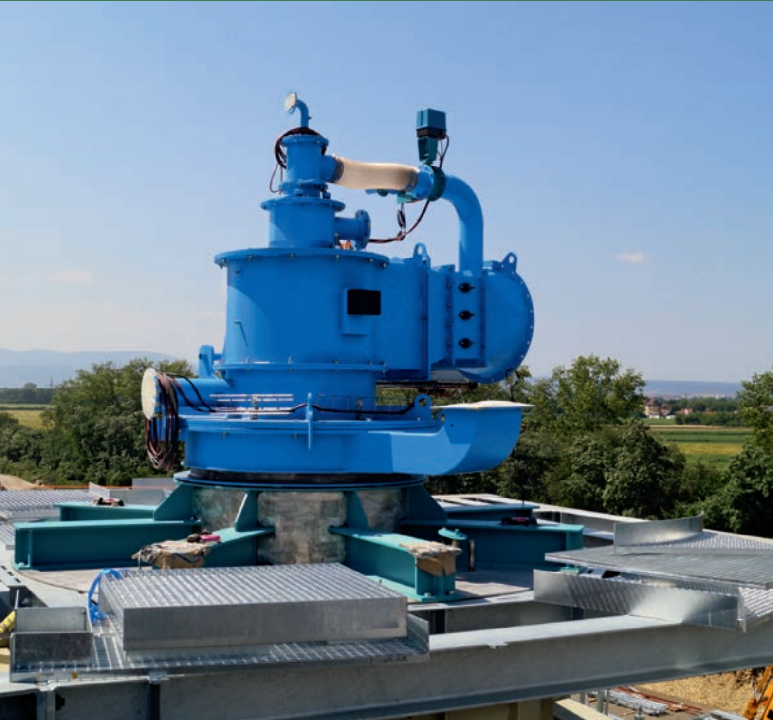
New Büttner BCB combination burner – Installation on the new vertical Büttner steel combustion chamber with no refractory lining
