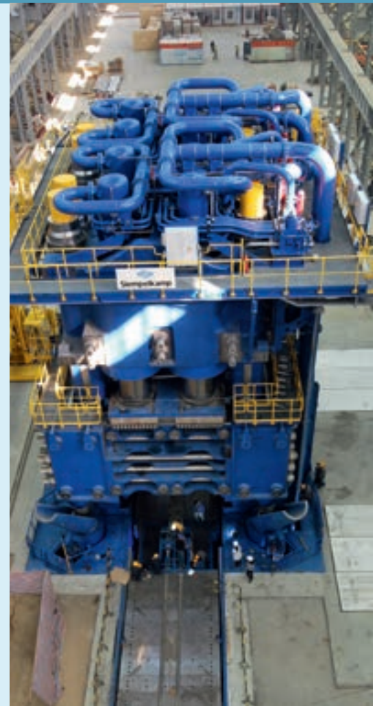
Hydraulic piping for the 8 press cylinders
