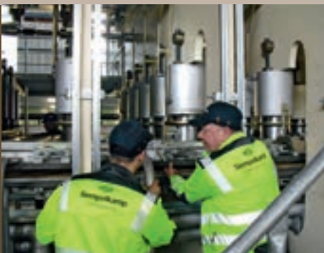
Service team in the field
