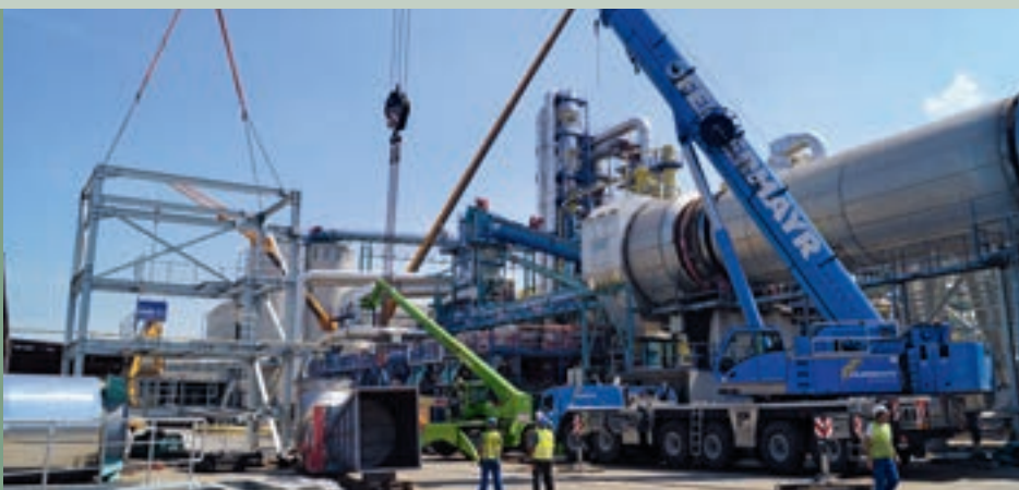
Steel structure for the new flash tube pre-dryer on the crane hook, ready for installation
