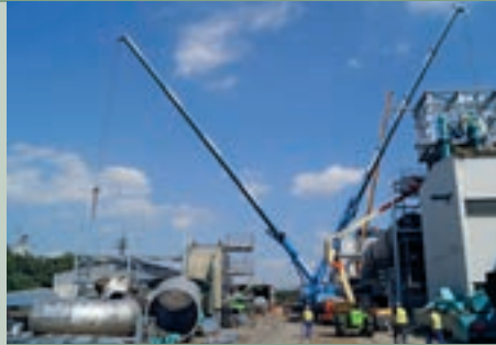
Two cranes in constant use – for a short modification phase. New components are preassembled, as much as possible, directly next to the dryer and immediately installed.
