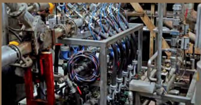
Ecoresinator for fibers during installation at Starwood
