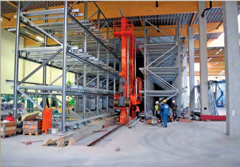
High-rack storage system for veneers
