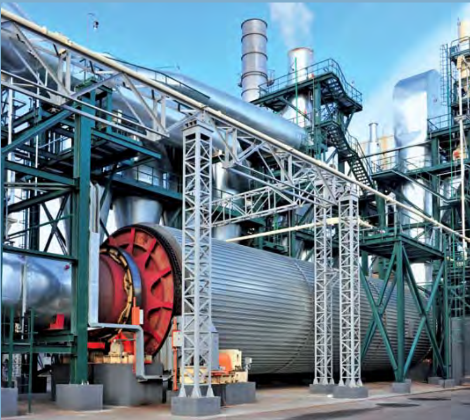
Complete provider of production plants for wood-based products, here: dryer and energy plant
