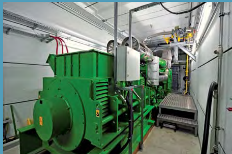
The engine inside the cogeneration unit
