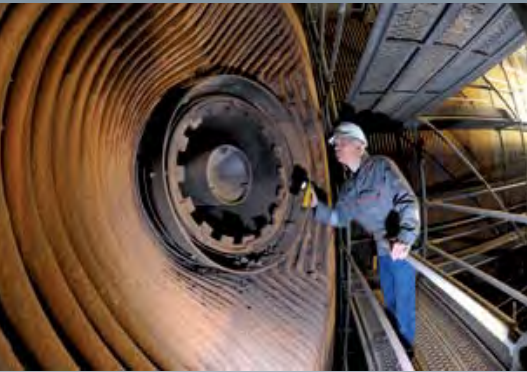
View into the burner of a boiler (photo: Andreas Seidel, Chemnitz)
