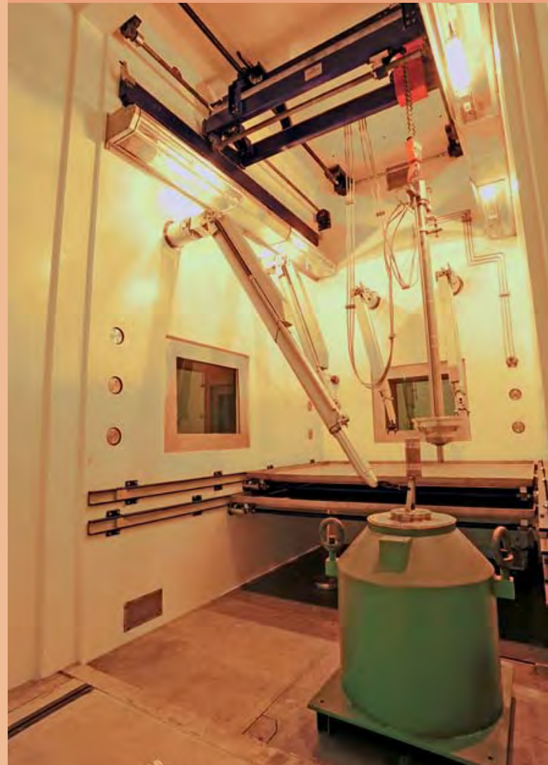
Interior view of the hot cell
