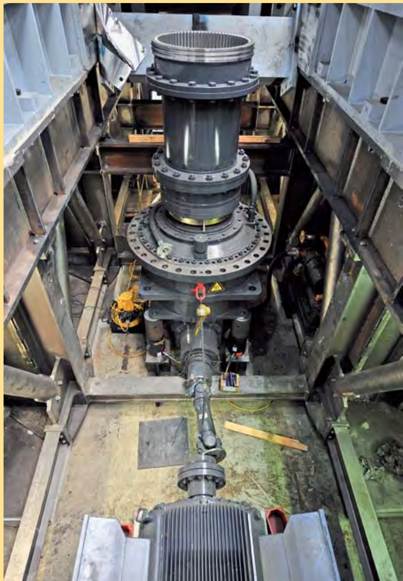
Motor and gear unit leading to the main roller shaft
