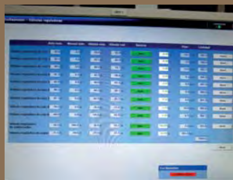
Flow display in the controller room
