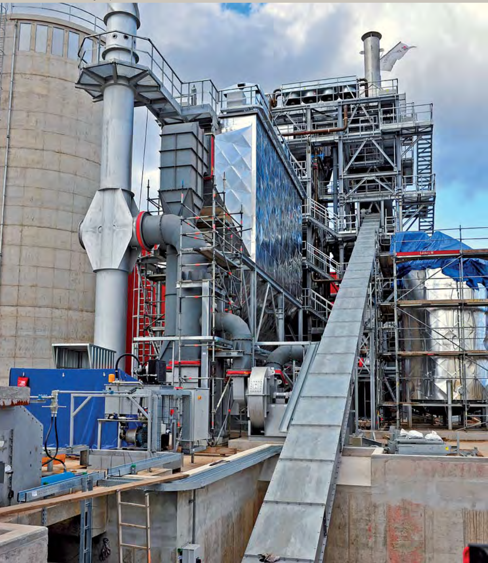
The 13 MW Büttner heating and power station
