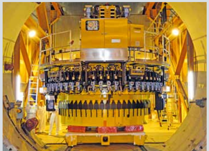
2011 at the Gravelines NPP: the new optimized Siempelkamp stud tensioner was delivered – insertion of the stud tensioner to the containment
