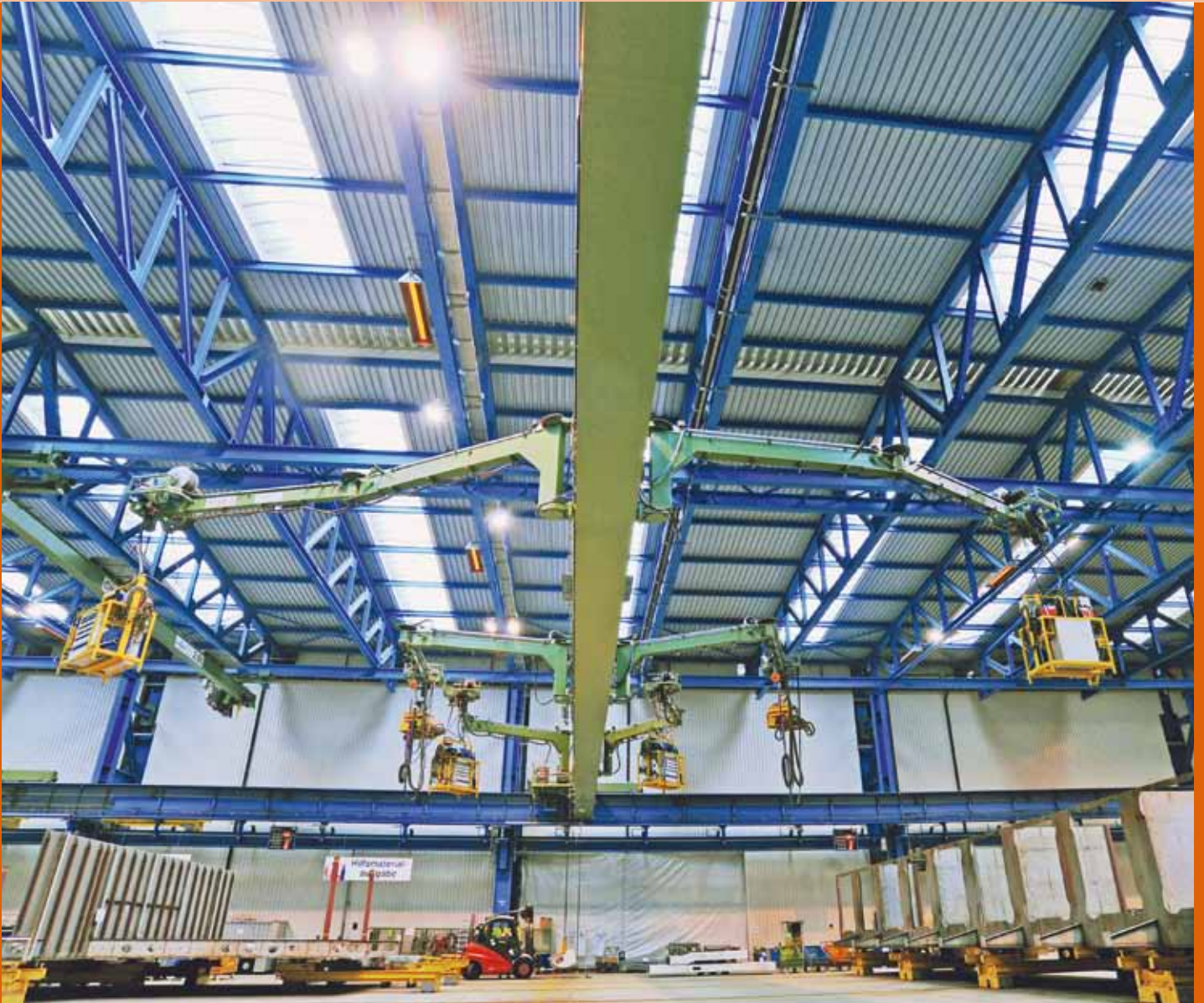
Single-girder bridge crane equipped with six knuckle booms and tool boxes
